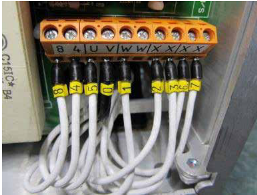
The picture shows 240VAC arrangement.
