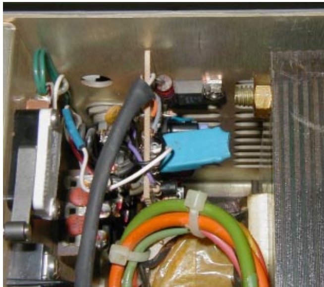
Photo 4. The board is installed on the rear panel between the power transformer and the tube compartment.
