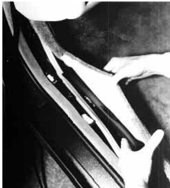
Figure 9 — Peel back the carpet in a Cadillac to permit a cable run
