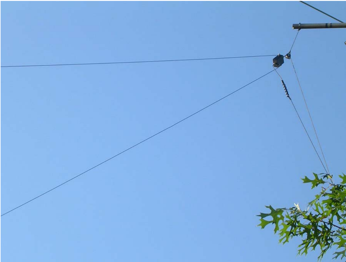
Feed point showing Balun hoisted into position on mast, Notice the strain relief for coax. Vee wires are pulled out taut to the ground rods.
