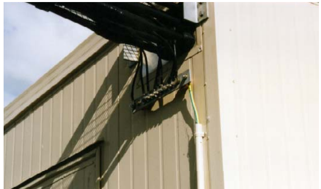
Figure 10. Cable sheath bonding at the building point of entry
