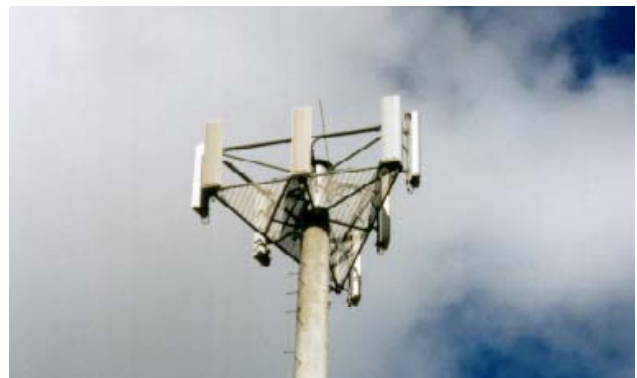
Figure 7. GSM antenna structure. Note lightning finial is of insufficient height.
